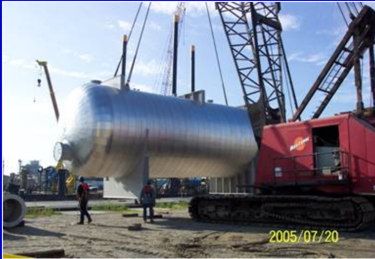
Oil Treater Vessel
